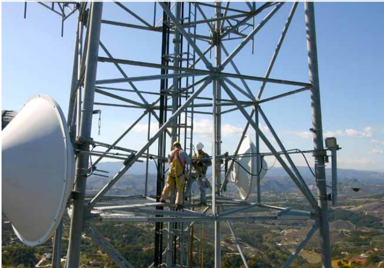
Pablo Bryant and Mark VanScoy, from San Diego State U, partnering with HPWREN on installation work at an HPWREN backbone site. Image credit: Hans-Werner Braun.
