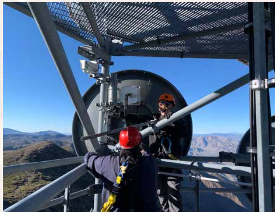
Following repair work, Jim Hale (front) and Adam Brust align an HPWREN antenna between Mount Laguna and the Palomar Observatory. Credit: HPWREN.
